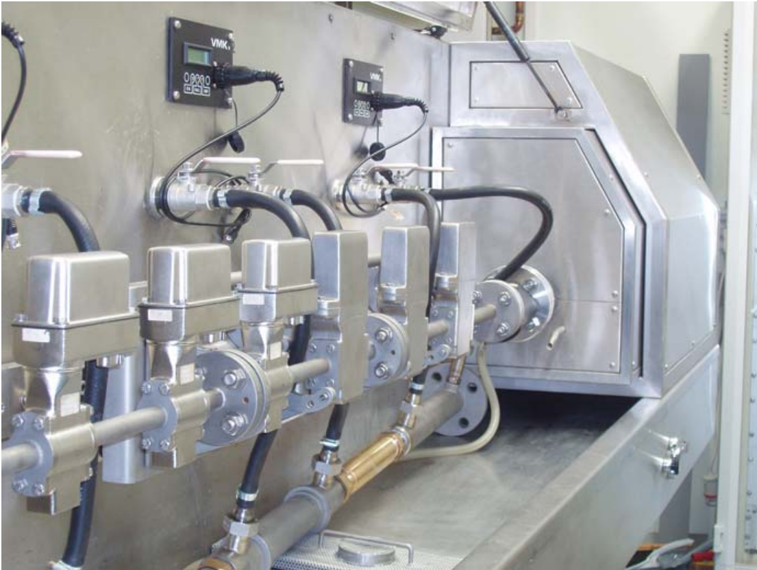
Fig.4 Installed MAGMETER in the PTB test section
