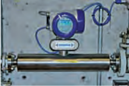
OPTIMASS 7300 with the tantalum measuring tube measures acidic solvents in a Swiss chemical company
