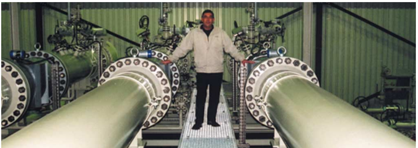
Zero maintenance and lowest cost of ownership. Triple bank of ultrasonic flowmeters
