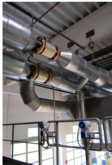
Hot water measurement in the boiler house at Krombacher
