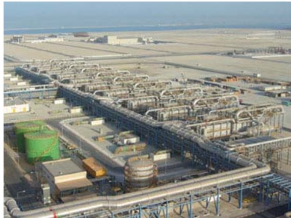
SIDEM desalination plant, Marafiq – Saudi Arabia
