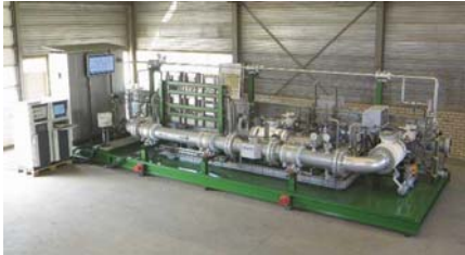
Flow Metering System
