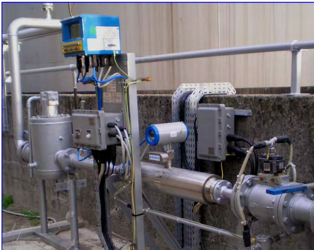
A fiscal metering station complete with air eliminator and a batch controller.
