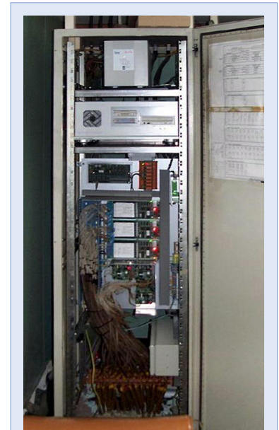
Existing cabinet with new electronics
